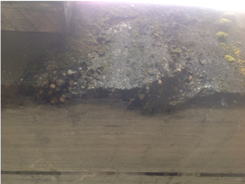
upstream slab damage
